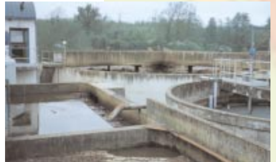
Diagnostic Station Epuration
